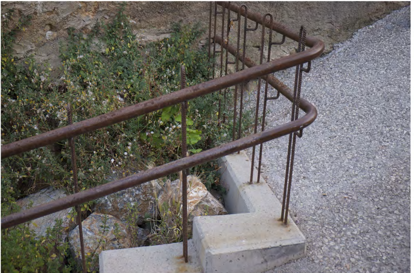
Turó de la Rovira, reinforcing steel as handrail. Photo: William John Maynard
