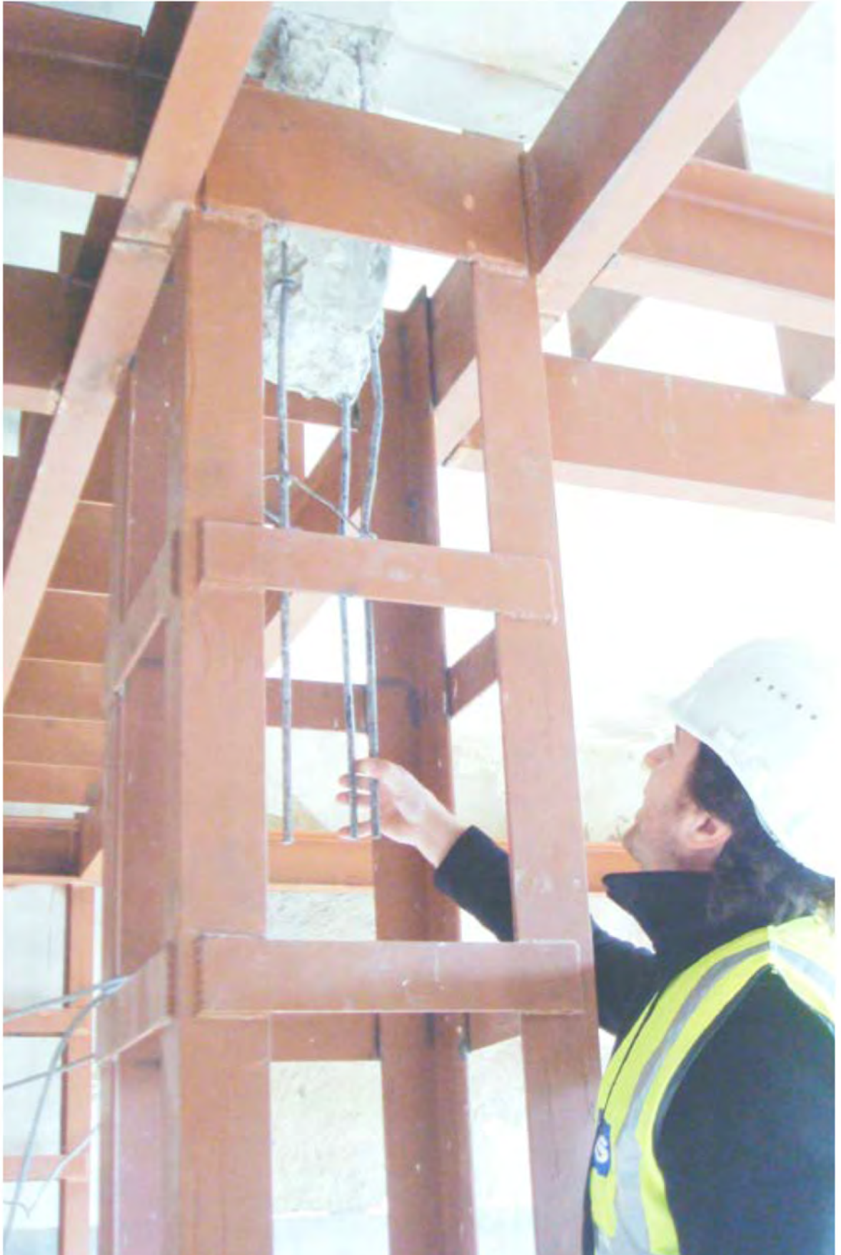
Engineering inspection of decayed column, Naves 8/9. Courtesy Arturo Franco.
