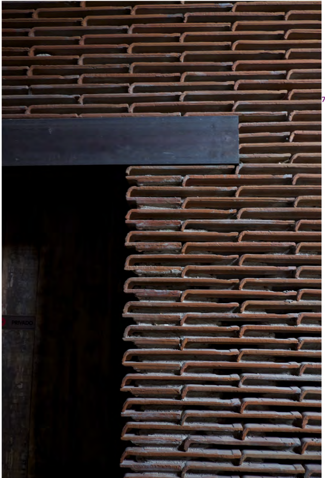
Entrance room with steel plate lintel, Nave 8b Arturo Franco. Photo: William John Maynard
