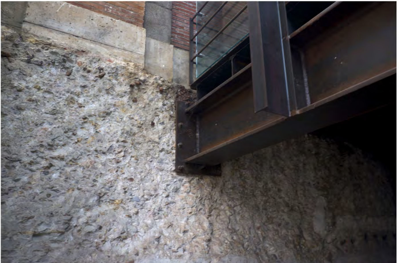
Mezzanine connection detail, La Aquirias, Héctor Fernández Elorza and Jesús Aparicio. Photo by William John Maynard
